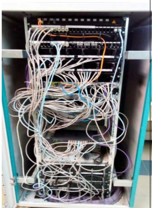
SG0046_RACK ZONA B AULA 2-12
